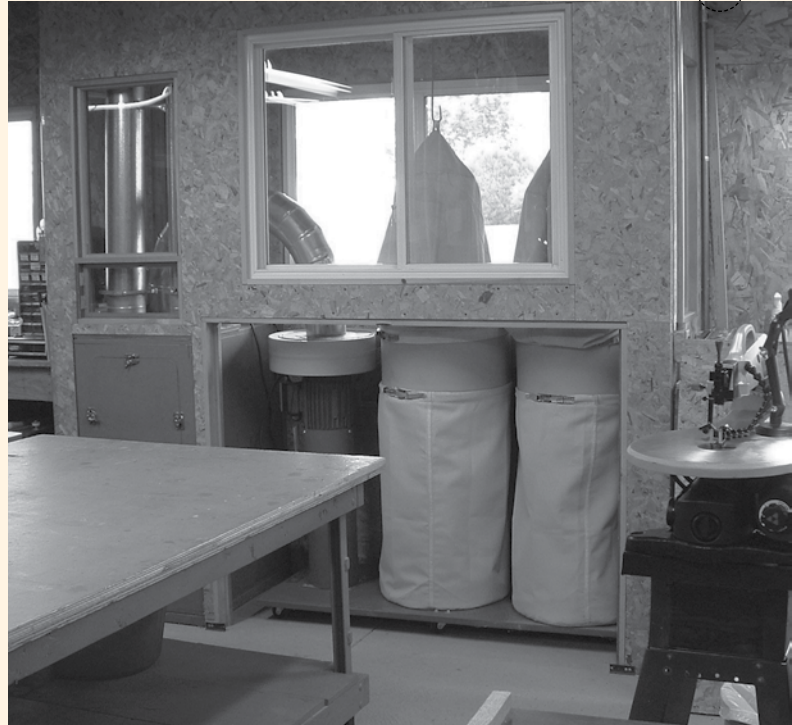
George Jaeger put his dust collection system in a bump-out along one wall of his Kentucky workshop. Windows let in the light and a removable panel gives him access for cleaning.
