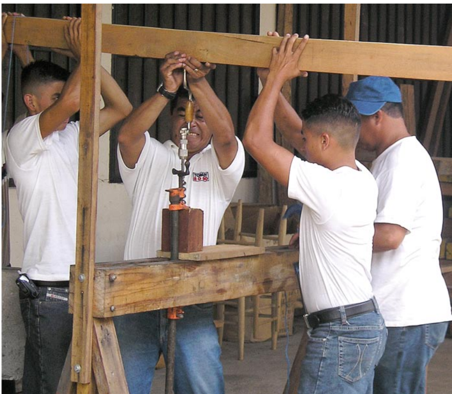
Old-fashioned ingenuity. The beam drill in action. The downward force provided by the beam above the brace assists greatly in boring accurate holes.
