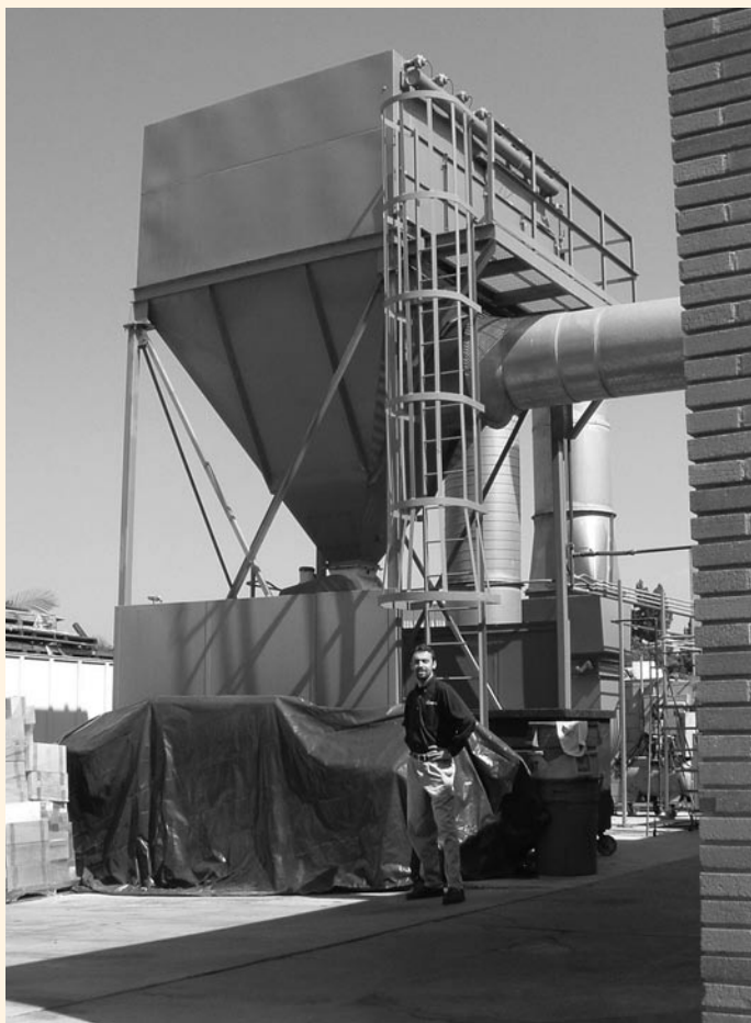
This gigantic dust collector services a big woodworking shop at Cerritos College in California. Small shops can use the same type of equipment – only a lot smaller in size.
