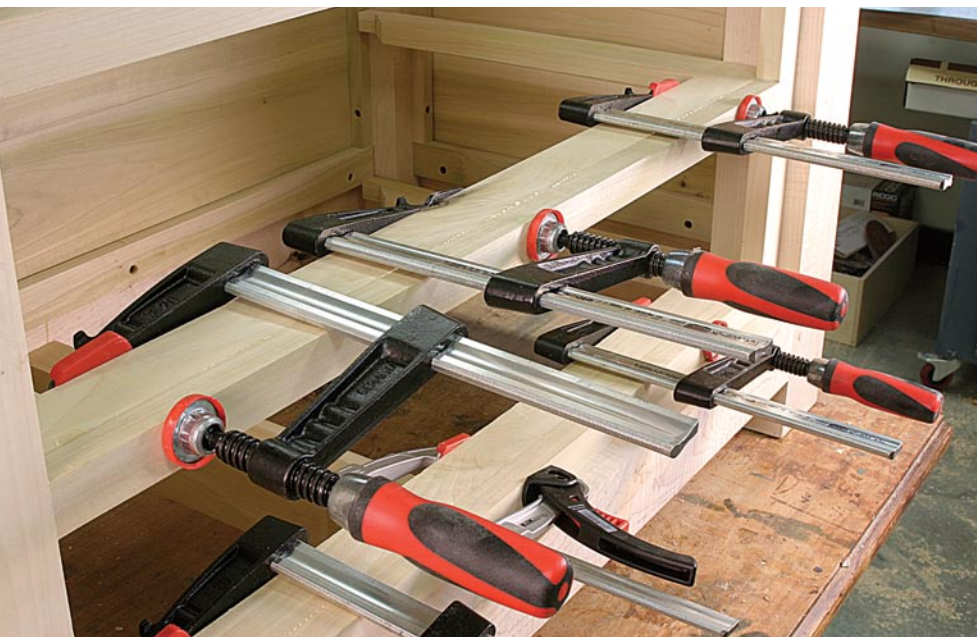
Clamps galore. Attaching the rail extensions to the face frame dividers requires many clamps. It's best to stage the process working one frame at a time. Once dry, level and nail the runners at the back.
